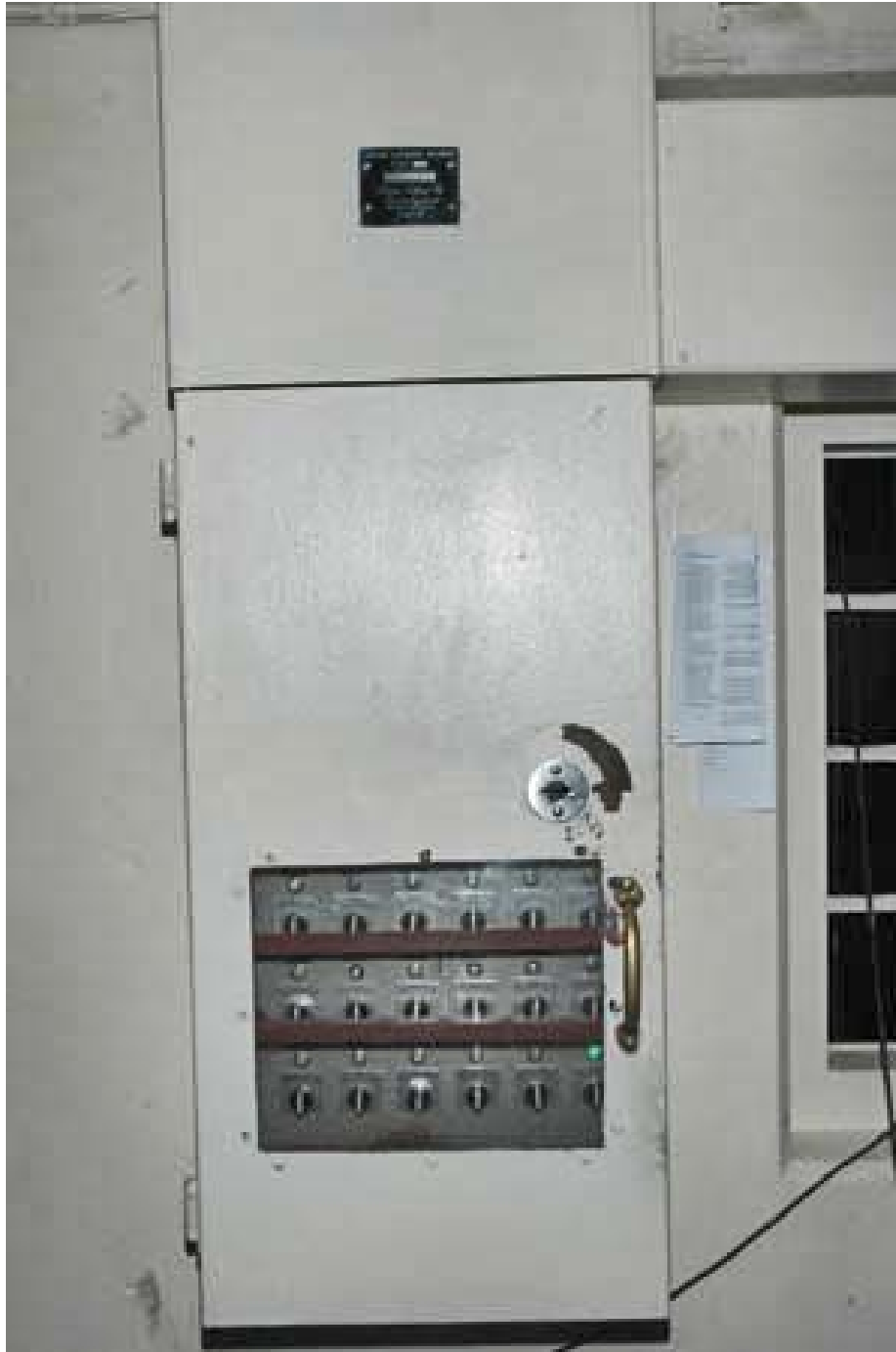
Controls for the Cell doors
