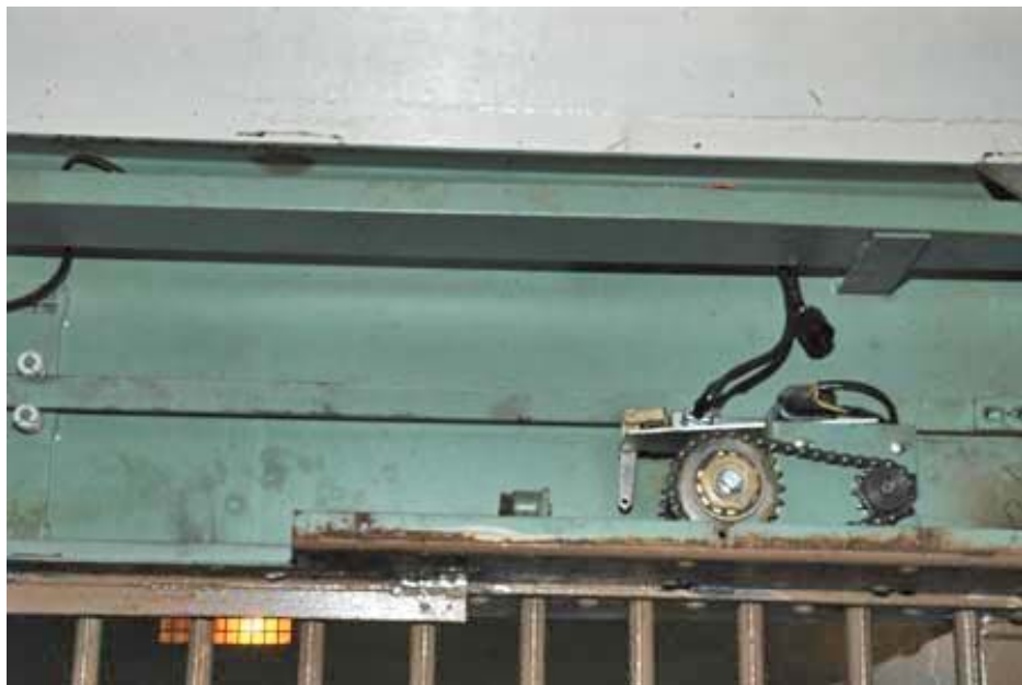
Interior of cell door mechanism
