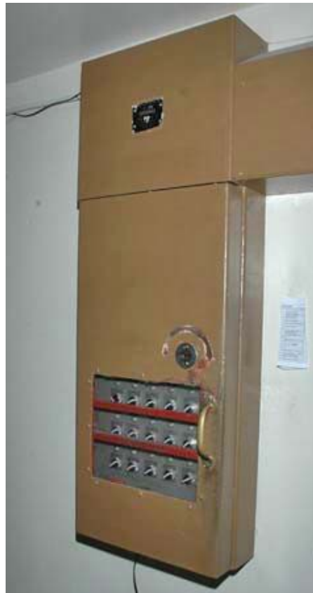
Cell door controls
